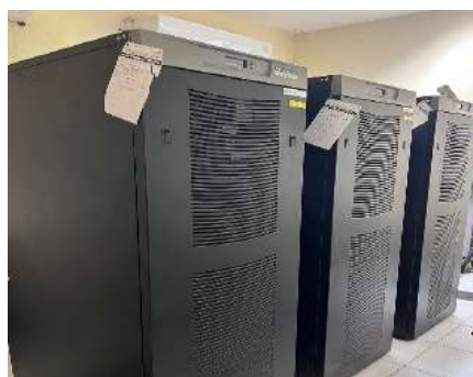
Gambar 7. Uninterruptible Power Supply Gardu Terminal
