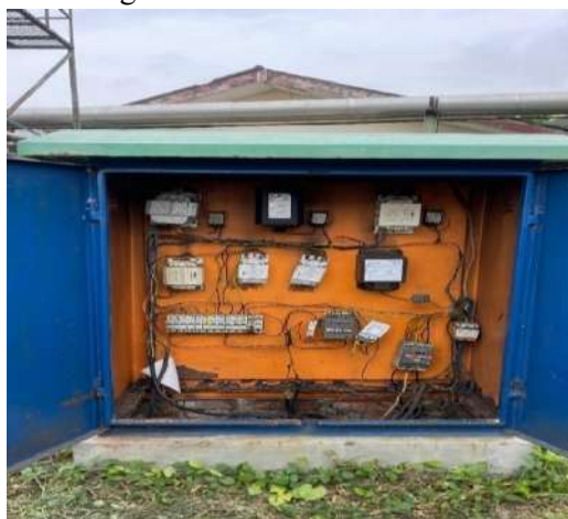
Gambar 3. Panel Lampu Floodlight Eksisting Sumber : Bandar Udara Internasional Halim Perdanakusuma
