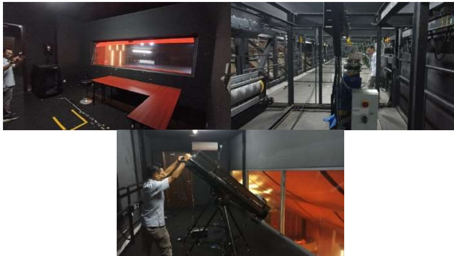
Gambar 7. Sound and Lighting control room
