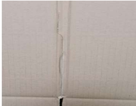
Gambar 1. Contoh Reject Cracking
